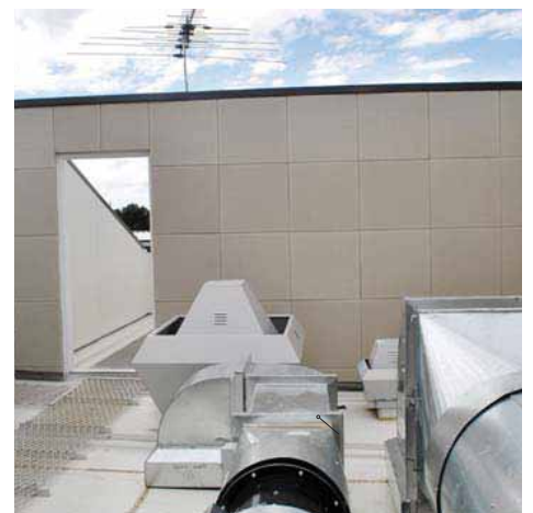
Cooling towers and HVAC
